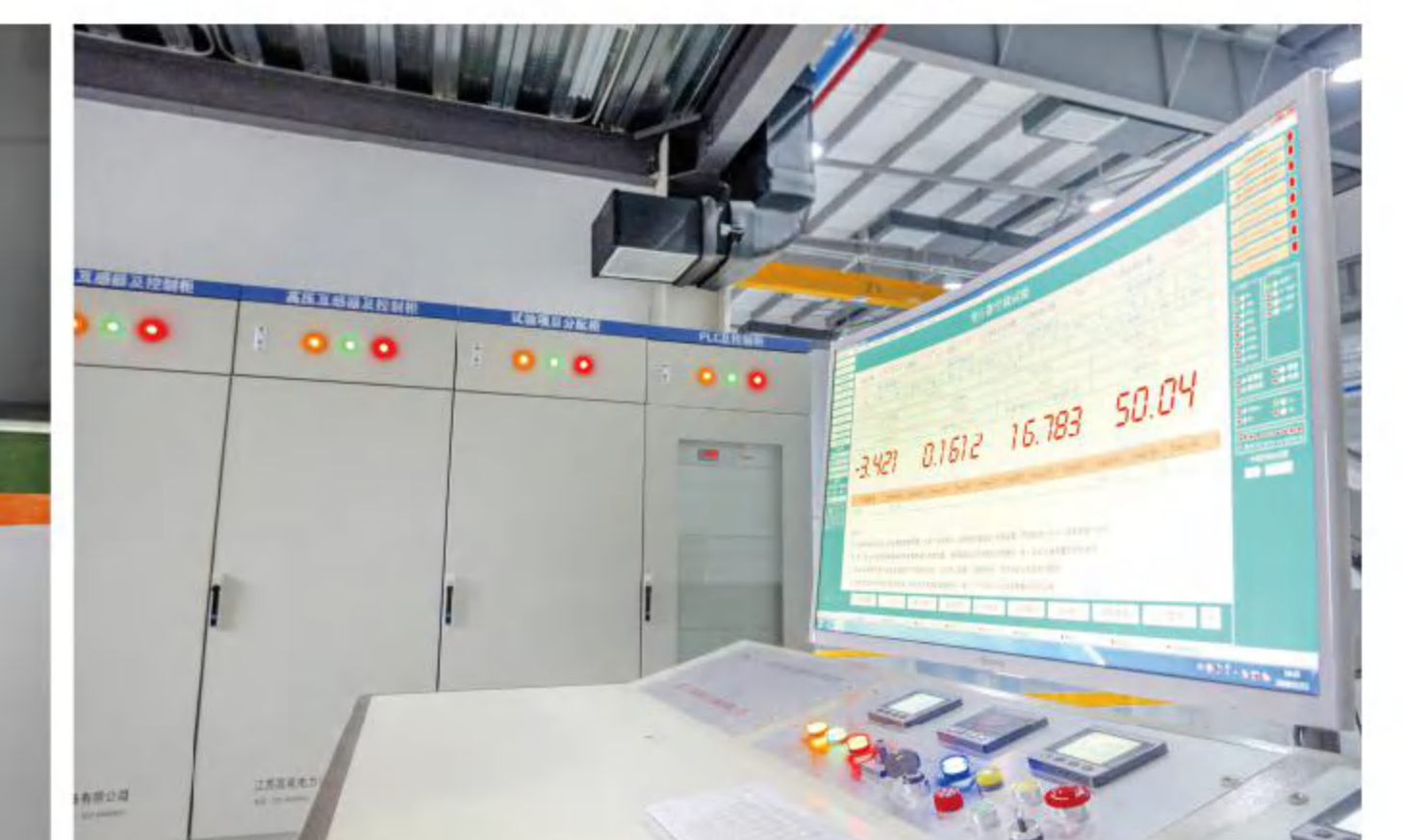
Transformer Core Integrated Test Center
